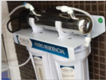
Water filters in each villa were renewed.
