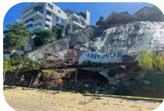
From the beach looking northeast; site of the landslide. Note the "rock-bolts" that have been installed on the left face of the site
