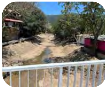
Nearly completed channel improvement work on the north side of the Isla Rio Cuale.
