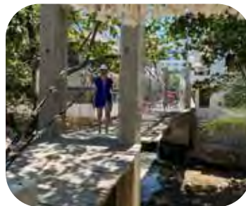
This is the newly rebuilt pedestrian suspension bridge across the south side of the river. Rebuilding of the northern suspension bridge is still underway.
