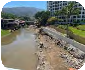
This is some of the work on the river's channel on the south side of Isla Rio Cuale. Oscar's restaurant is on the left. This picture was taken from the pedestrian bridge over the Rio Cuale on the Malacon
